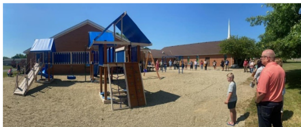
We installed a brand new playground for the community to use and demolished the old dangerous equipment.
